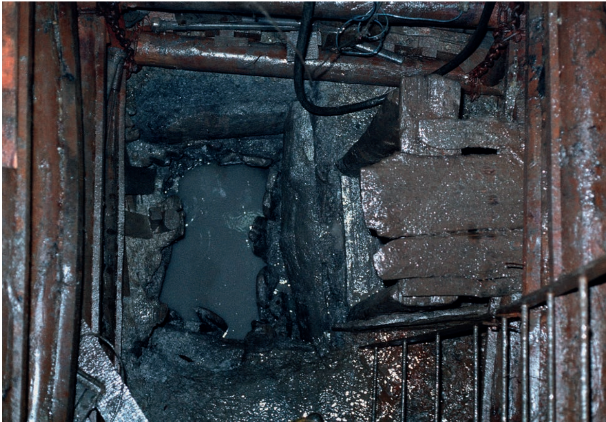
Figure 3: Original medieval Shaft 2 with connecting medieval gallery. The medieval shaft was followed and expanded during later mining. Photo: P. Thomas, DBM.
